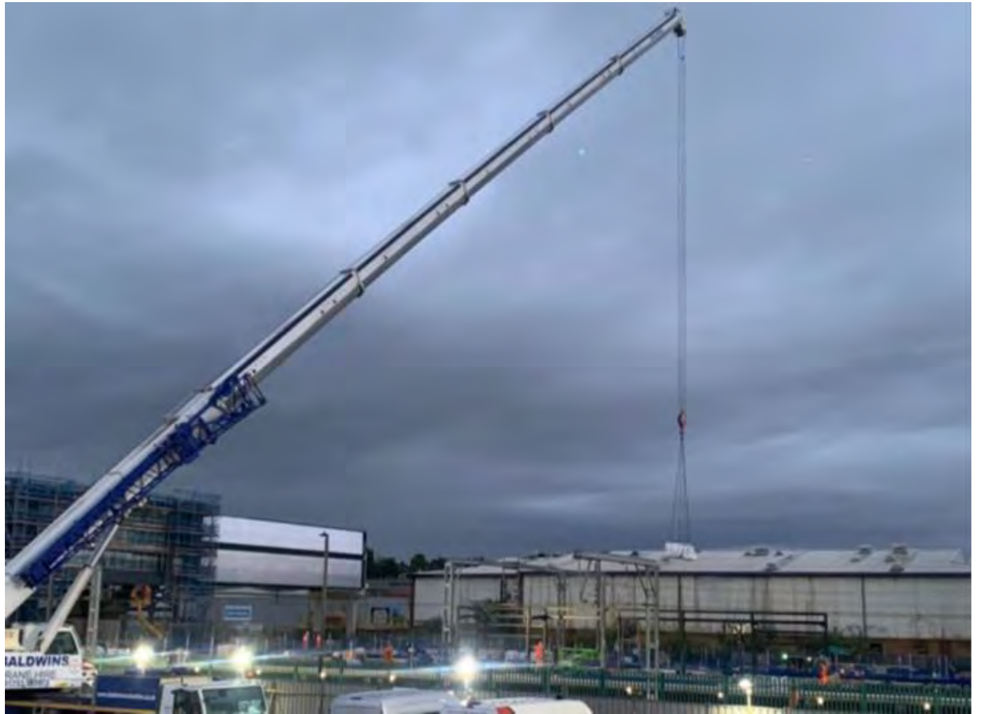
Steel lifts for the platform waiting rooms
